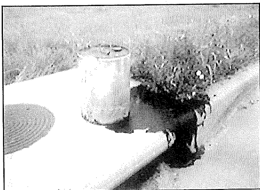
Figure 5: Dumping at a storm drain inlet
